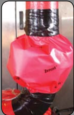
Offshore Platform Fire Water Line
