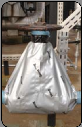
Coastal Terminal Oil line with Gate Valve
