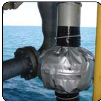
Offshore Platforms & Rigs
